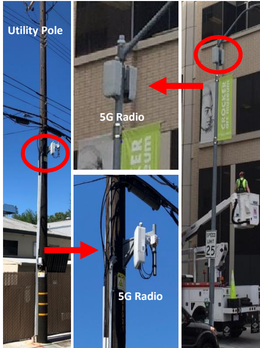
Sacramento (Utility & Light Pole)
